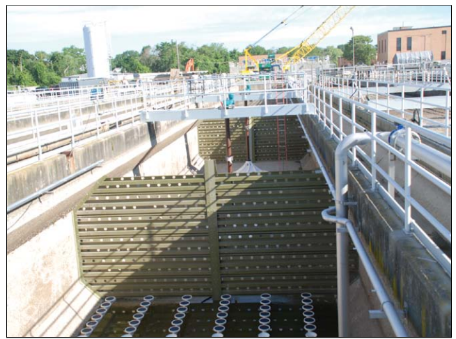
Figure 1. Stratford aeration tank.
